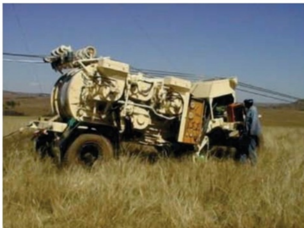
Typical example of tensioner station
